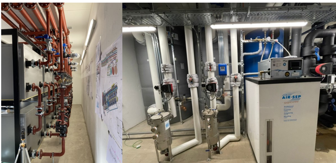
Figure 5 – The skid mounted heat pump modules at the swimming pool.
